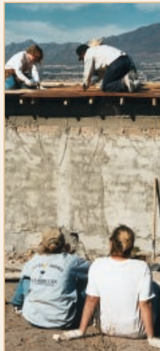
Two-ply boards are used for the first layer of the roof, followed by tar, tar paper and shingles.
