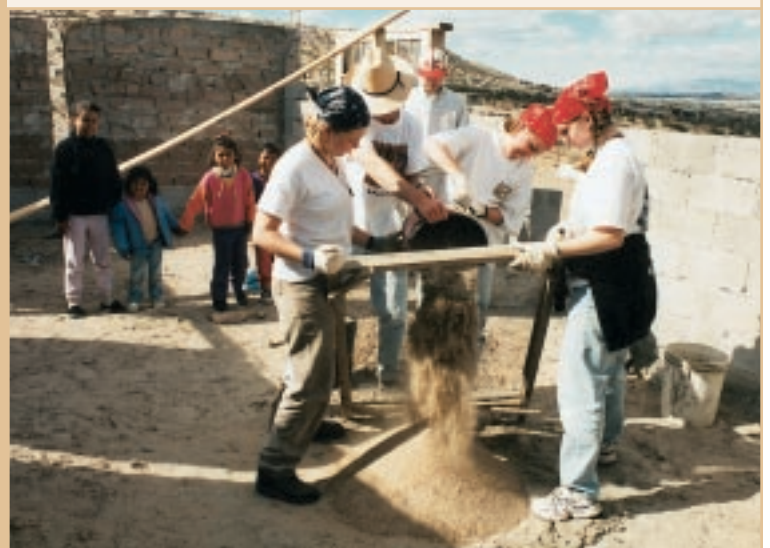
Sand is carried by truck from the hillside outside of town and strained in preparation to make cement.
